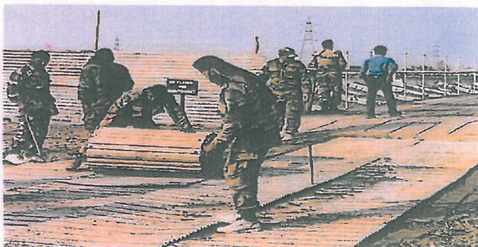
Photo - 1: Laying of Pontoon bridges across Yamuna by trained professionals note the ramps are made-up of wooden 'approach slab' and corrugated metal sheet and not of debris and stone grit as claimed by the Principal Committee.
