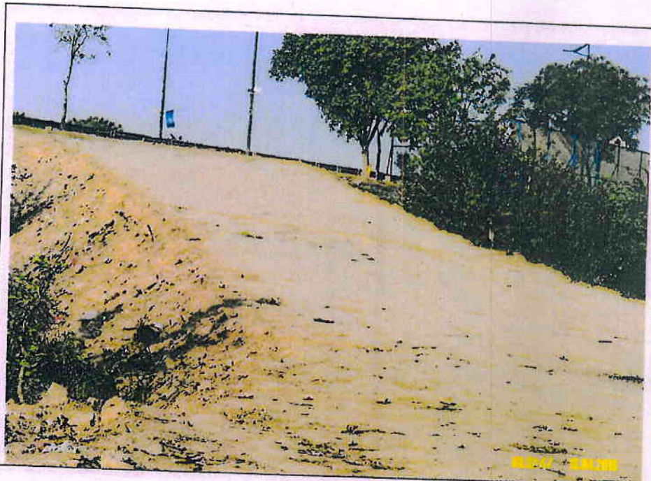
Photo - 1: One of the three earthen ramp constructed over the embankment of DND Flyway for World Culture Festival 2016
