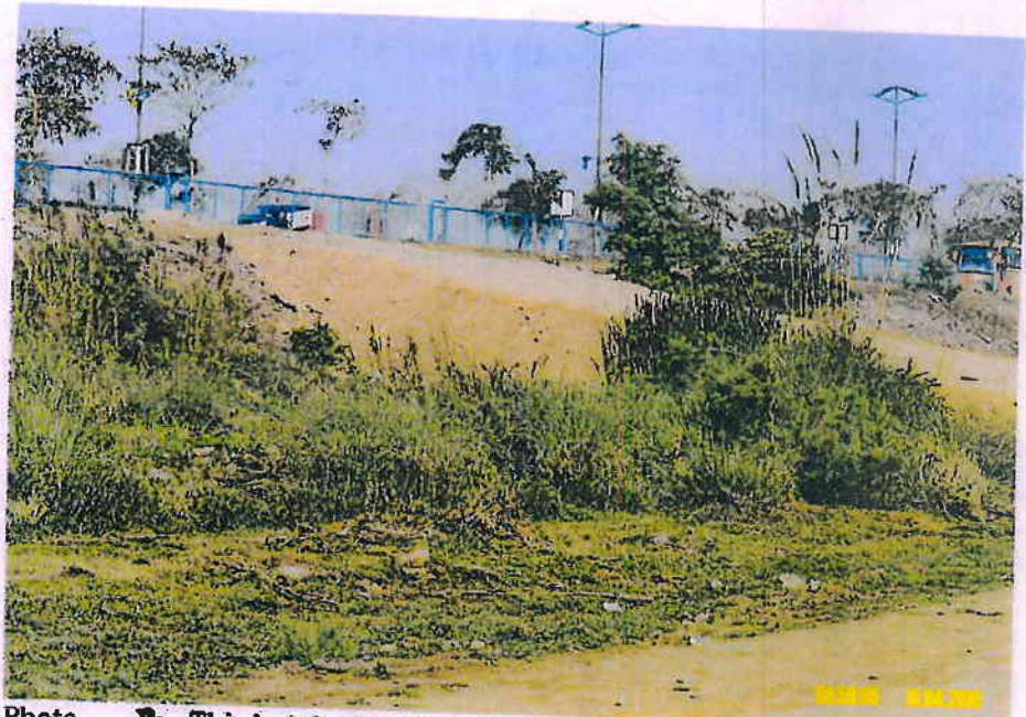
Photo - 3: Third (of the three) earthen ramp constructed over the embankment of DND Flyway for World Culture Festival 2016
