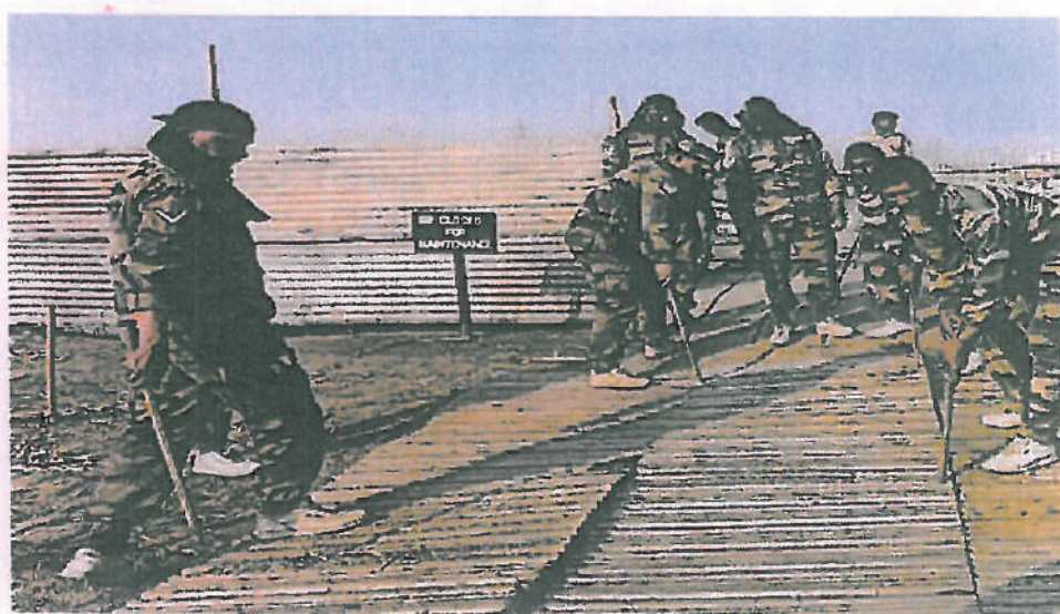
Photo - 2: Laying of Pontoon bridges across Yamuna by trained professionals note the ramps are made-up of wooden 'approach slab' and corrugated metal sheet and not of debris and stone grit as claimed by the Principal Committee.
