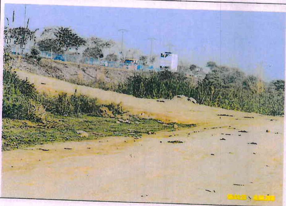
Photo - 2: Second (of the three) earthen ramp constructed over the embankment of DND Flyway for World Culture Festival 2016
