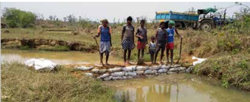
Guided by Yuvacharyas, villagers construct a simple check dam in a stream bed
